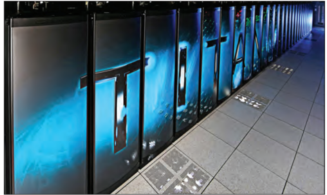
Titan supercomputer (Oak Ridge National Laboratory)
