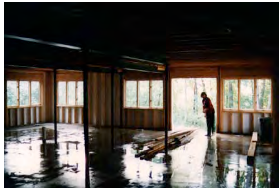
And the basement floods
