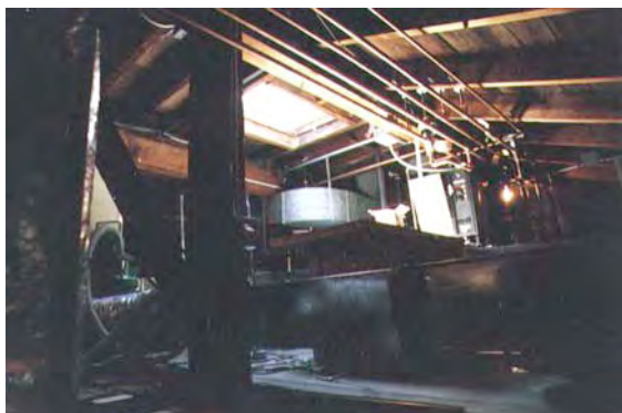
An industrial-grade HVAC system
